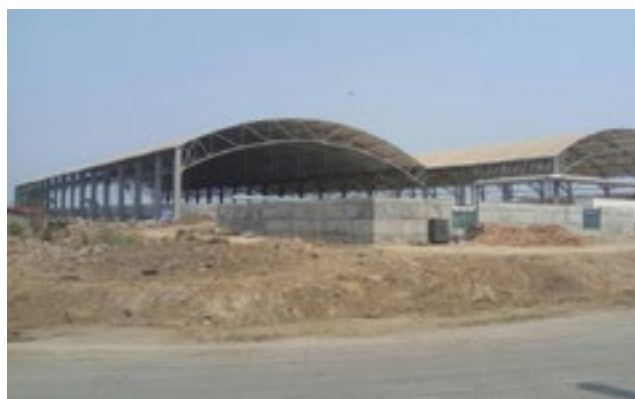
Municipal Solid Waste Treatment Plant in Mumbai, India
